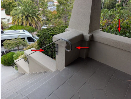
Low guardrail, large openings, and non-returning handrail
